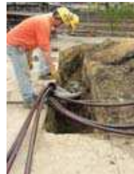
Underground transmission system.
