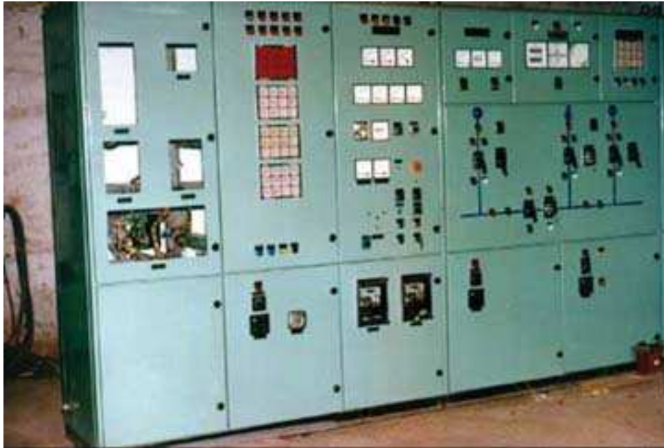
Power Factor Improvement
