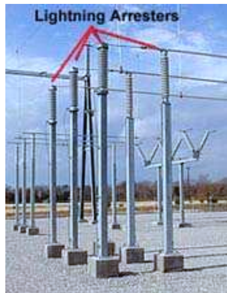
Lightning arresters on bus structures
