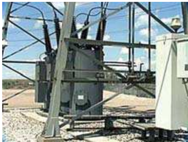
Oil circuit breaker
